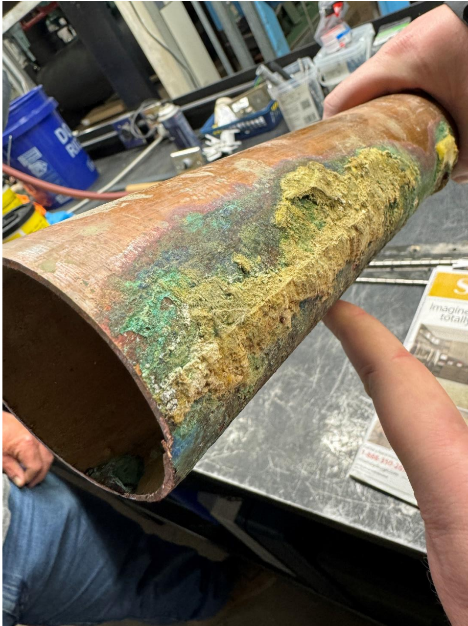
Image 2: Typical Corrosion of the Domestic Water Piping System
